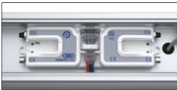
Power supply is connected
